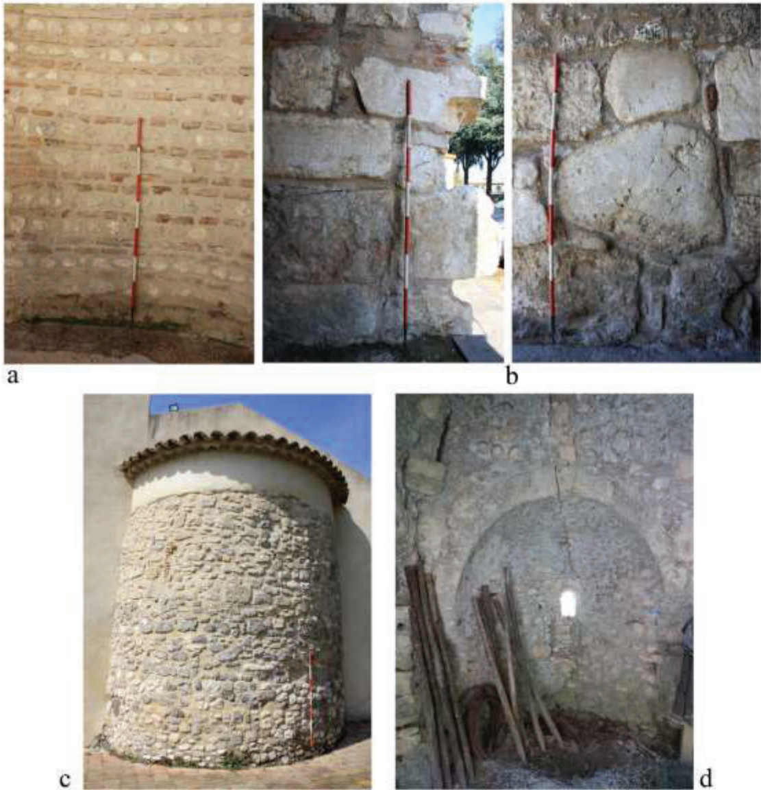
Fig. 4 - Some examples of masonry techniques: S. Maria di Compulteria, opus listatum (a) and big blocks technique (b); “opera incerta” in S. Andrea di Marafi (c) and Campo la Fontana (d) (author’s photos).
